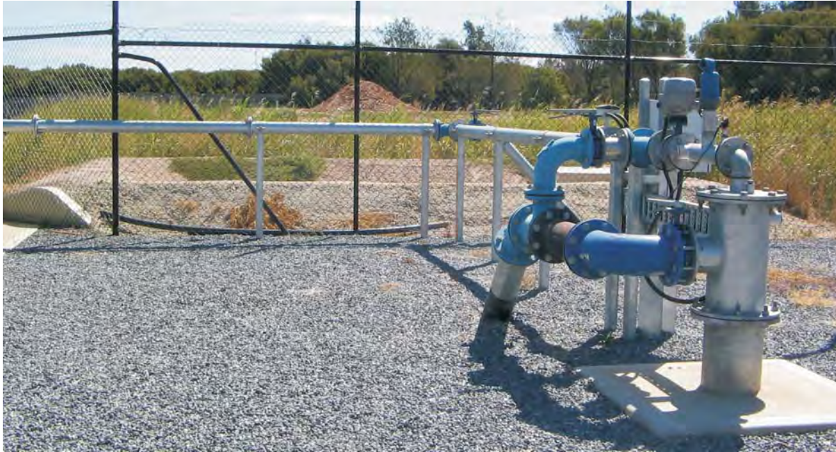
ASR headworks, Greenfields.
